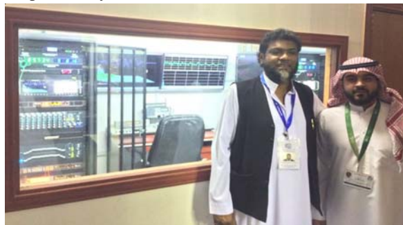
Photo above from left: Shaikh Shafayat and Bro. Rizwan standing in the control room.
